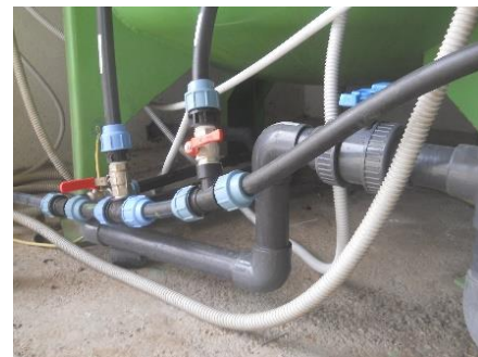
Figure 4: Pipeline for fertirrigation.
